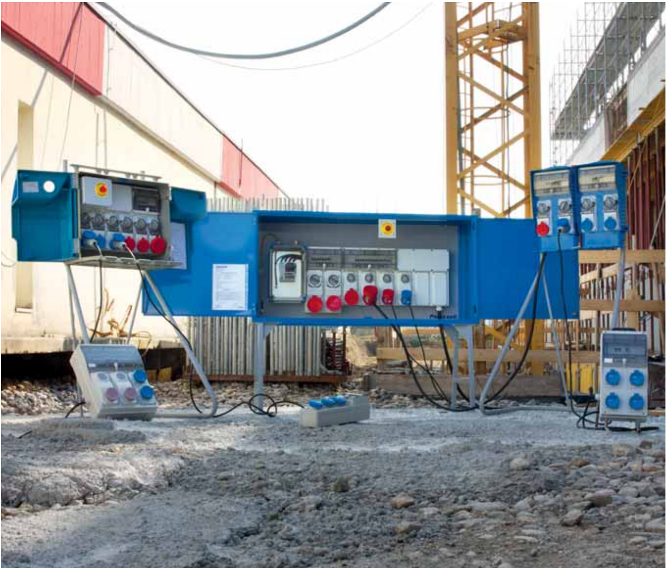
DISTRIBUTION AND TRANSFORMATION ACS BOARDS
